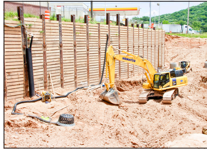
While work appears to have slowed down on the sinkhole repair, GDOT assures the public that construction continues apace. Photo by Shawn Jarrard
